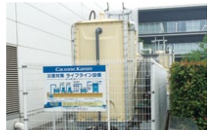
Groundwater membrane filtration system
