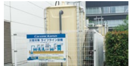
Groundwater membrane filtration system installed at the R&D Center and Headquarters
