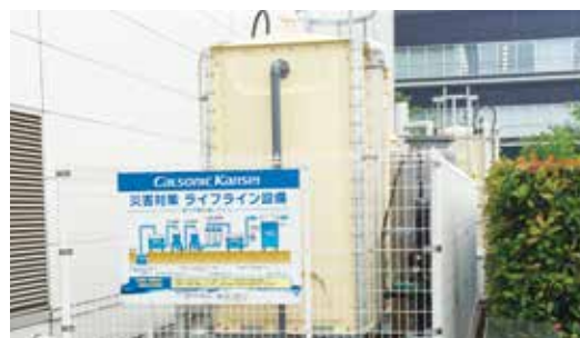
Groundwater membrane filtration system
